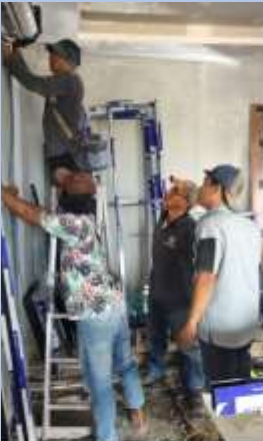
Test drain AC area Aula lt. 1
