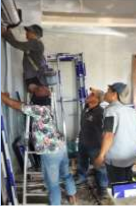
Test drain AC area aula lt. 1
